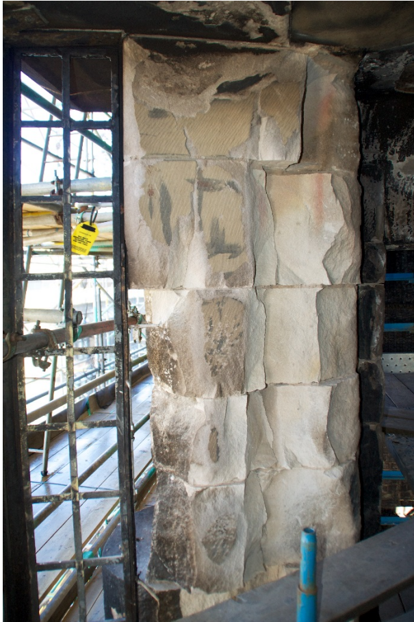
4. Loss of masonry of the library piers
